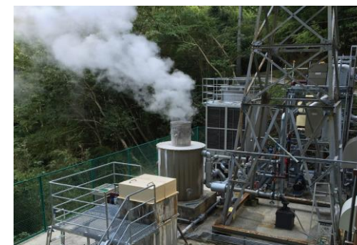
Shimoda Onsen Binary Power Plant
