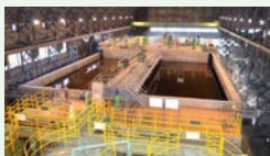
Motoyama AMD treatment facility at Toyoha Mine
