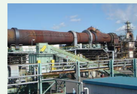
JX Nippon Tomakomai Chemical rotary kiln furnace
