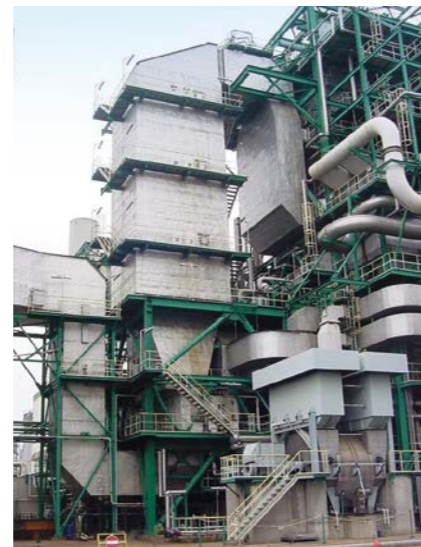
Flue gas denitrizer
