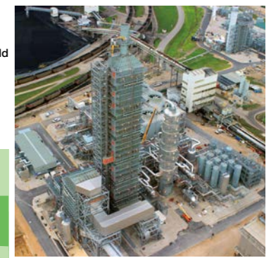
CO 2 recovery plant (state of Texas in the United States)
