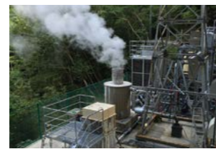
Shimoda Onsen Binary Power Plant
