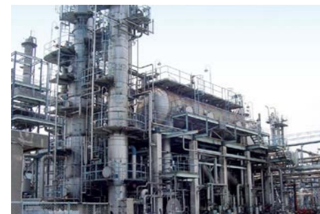
Sulfur recovery unit
