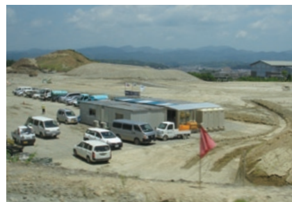
The planned site of a pressing and plating plant. (Kakegawa City, Shizuoka Prefecture)
