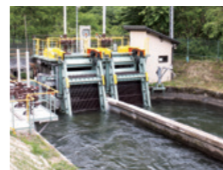
Kakinosawa Hydropower Plant
