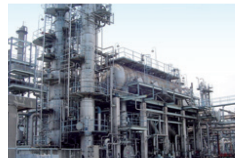
Flue gas desulfurizer
