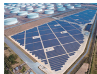
Uruma Mega Solar Power Plant
