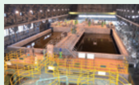
Motoyama AMD treatment facility at Toyoha Mine
