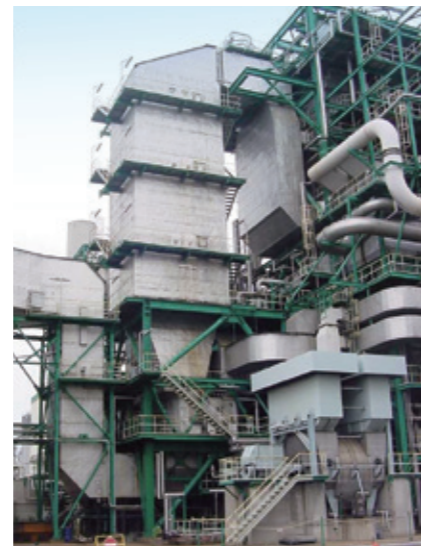
Flue gas denitrizer
