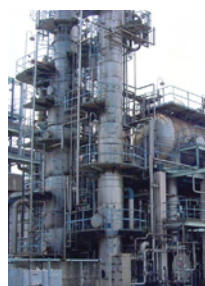
Sulfur recovery and flue-gas desulfurization equipment at the Mizushima Oil Refinery
