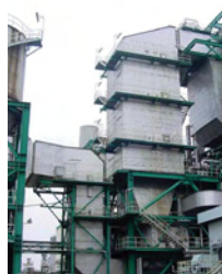
Flue-gas denitration equipment at the Mizushima Oil Refinery
