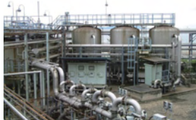
Wastewater treatment facilities that use activated carbon absorption
