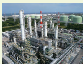
Sulfur-free gasoline production facility at the Mizushima Oil Refinery
