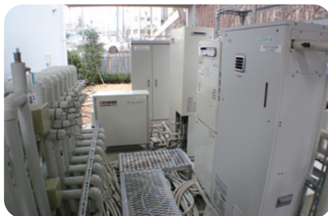
Energy devices installed at SOENE House (from left: ECO-FEEL, ECO-JOZU, ENE-FARM)
