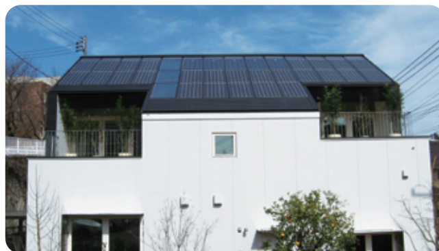
Solar power and water heating systems installed on the southern side of the roof
