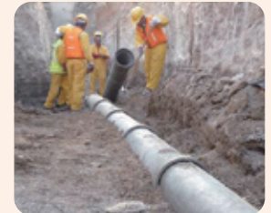
Recosul sewer pipe
